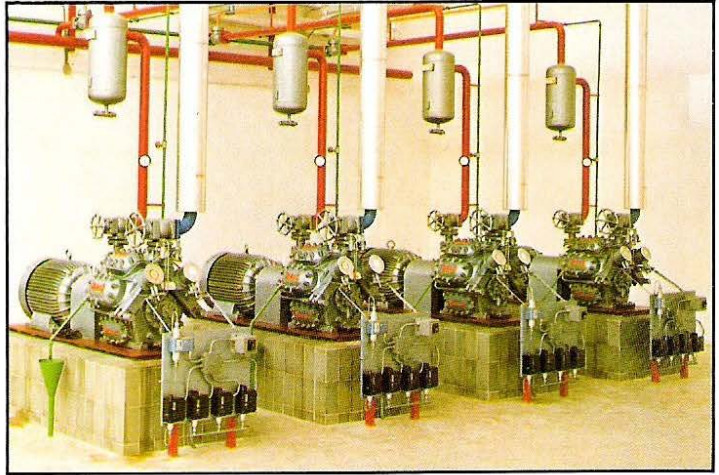
Fish industry in Spain with HC 8-75 compressors.
