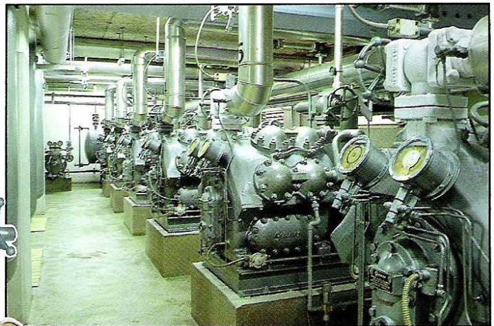
HC-800 compressors in a Danish slaughterhouse.
