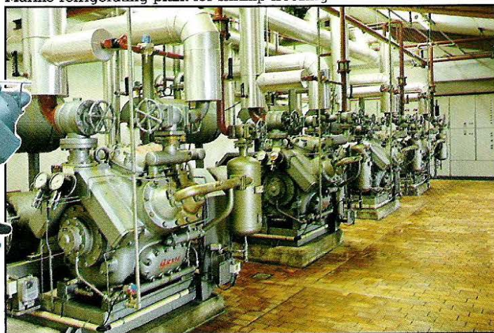
Fish freezing plant with HCT-125.
